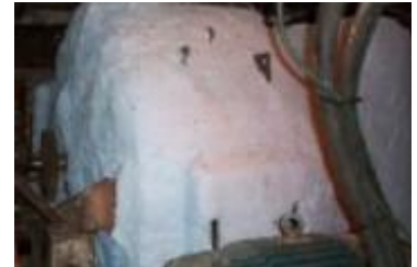
AI - Soaking Pit Fan Housing
